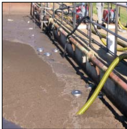
➤ Sewage tank during skimming cycle
