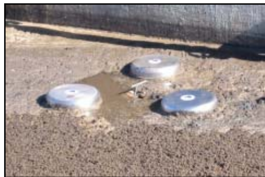
⊖ Sewage scum removal
